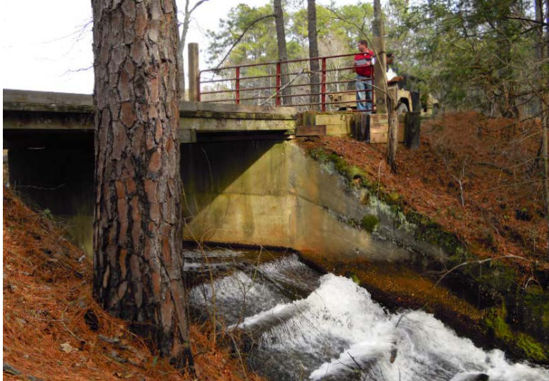
Figure 10. View of the downstream spillway wingwall on the east side of the dam. The seam between the ca. 1936 spillway and the newer ca. 1960 alteration is evident.
