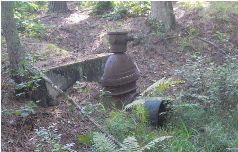
Figure 11. The dam's low-level outlet is located to the east of the principal spillway.
