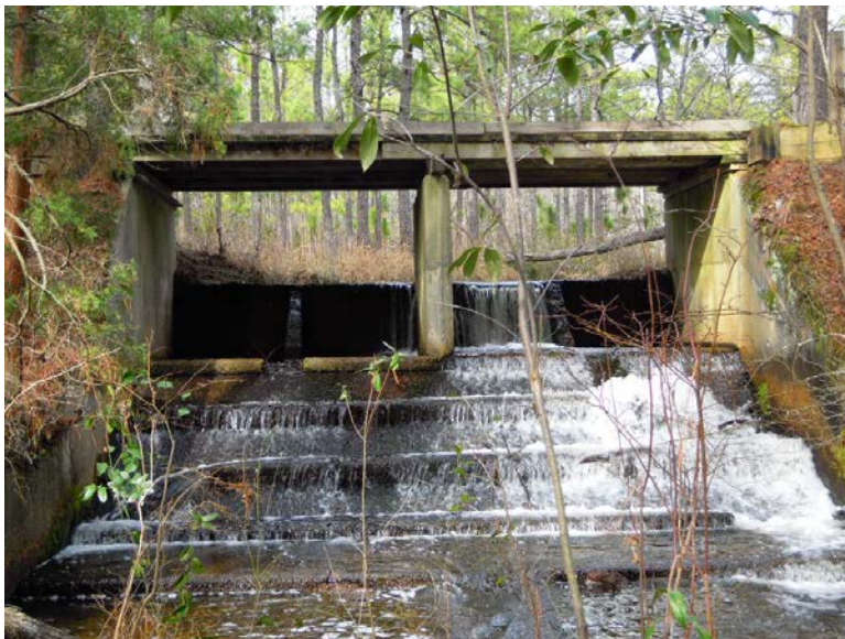
Figure 9. View of the spillway from downstream. Note the defined line running horizontally on each of the spillway walls and the center pier, separating the older concrete spillway, from the ca. 1960 concrete addition, built to raise the road and support the bridge across the spillway.
